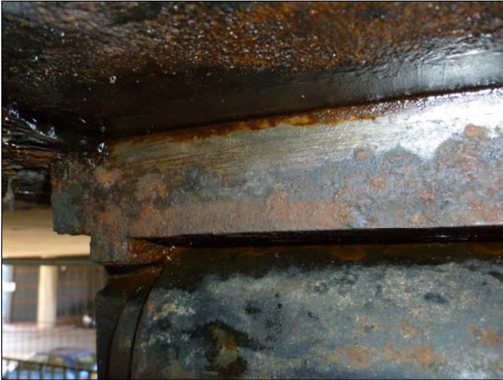
Bearing A2; Surface corrosion along front face of top plate.
