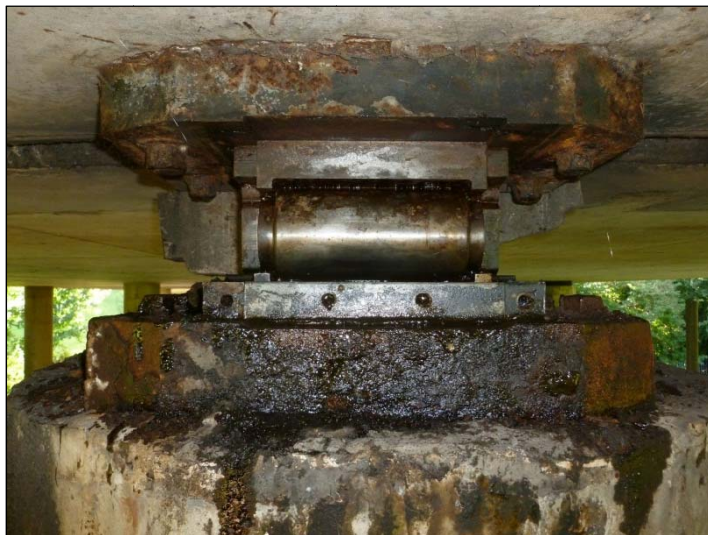
Bearing C1 with Grease Box Removed
