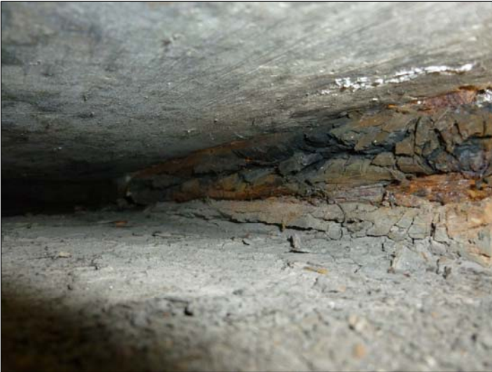
Bearing A; Cracking to elastomer and corroding steel plates.
