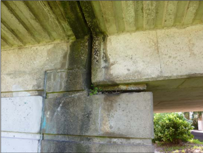
West End of Abutment, Adjacent to Bearing D; Heavy water staining around and below the joint.
