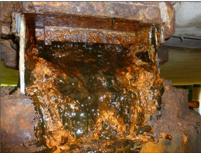
Bearing D2, There was a large amount of water came out of bolt holes of the grease boxes upon removal at C2 & D2. Here at D2 to you can see the condition of grease upon the removal of the box.
