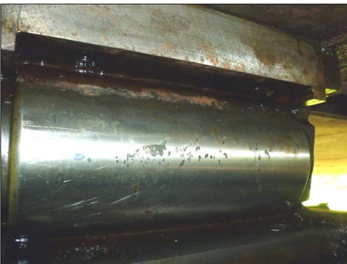
Bearing C2; Typical condition of rollers at pier 13. Minor surface pitting is common across the surface of the rollers.
