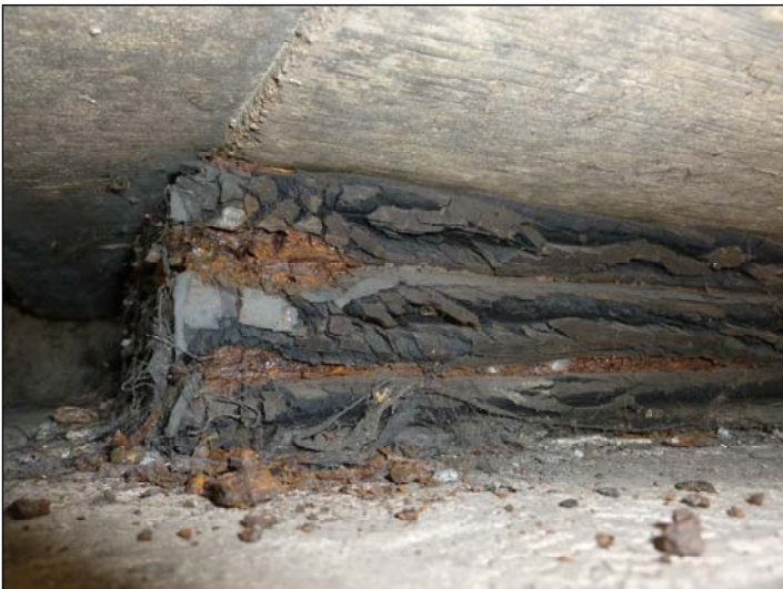
Bearing D; Deterioration to the elastomer and corrosion to exposed steel plates.
