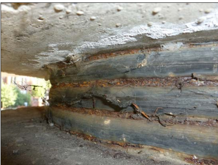
Bearing B; Deterioration of bearing exposing corroding steel plates.
