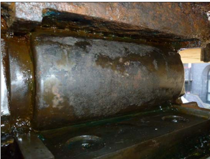
Bearing C1; Surface corrosion over large area of roller.
