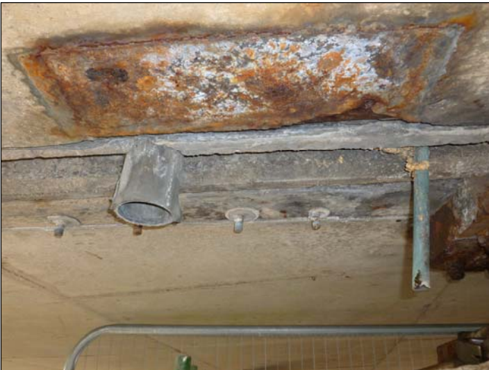
Adjacent to Bearing C1 & 2 One corroding steel plate has been left attached to the deck soffit adjacent to deck edge but similar plates have been removed from along the rest of the deck edge.
