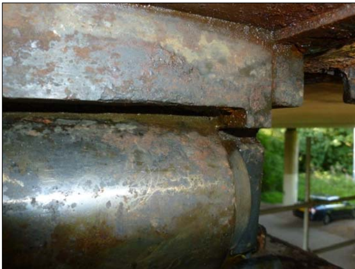
Bearing A2; The roller to bearing A2 is in the worst condition of the 8 at pier 13. There is more pitting to the surface and surface corrosion mostly across the top of the roller, this may be due to reduced cover from grease. Also note the surface corrosion to the top plate.
