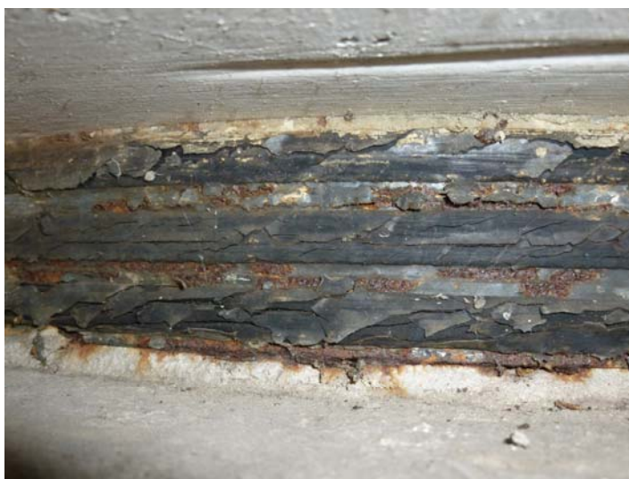
Bearing B; Deterioration of elastomer, exposing steel plates which are corroded.
