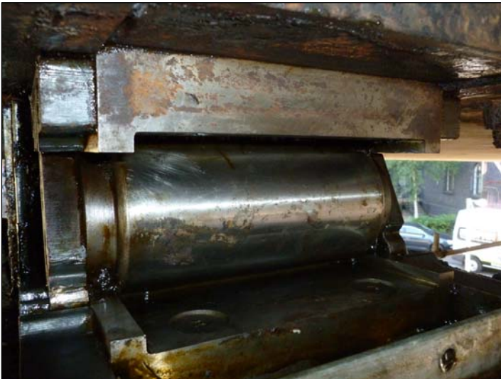
Bearing B1; Roller to bearing B1 however is in good condition with minor pitting to surface.
