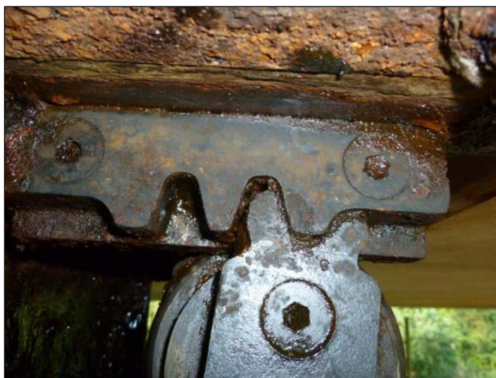
Bearing A1; Pitting and surface corrosion is common to the upper elements of the guide arrangement. Also note how the roller guide has been set on the wrong tooth.
