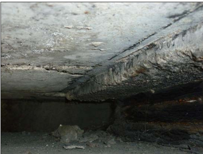
Adjacent to Bearing A; Delaminated concrete to the deck soffit and top plinth of bearing A adjacent to the deck edge.
