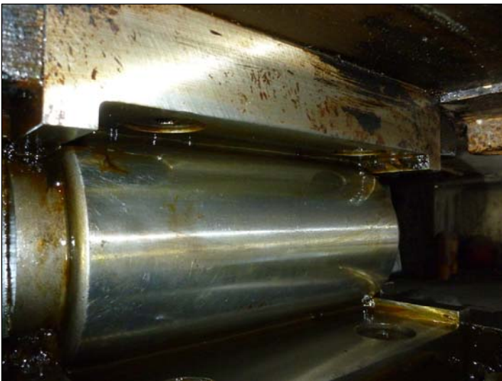
Bearing B; Typical condition of the Ashmead Way abutment bearings are very good.
