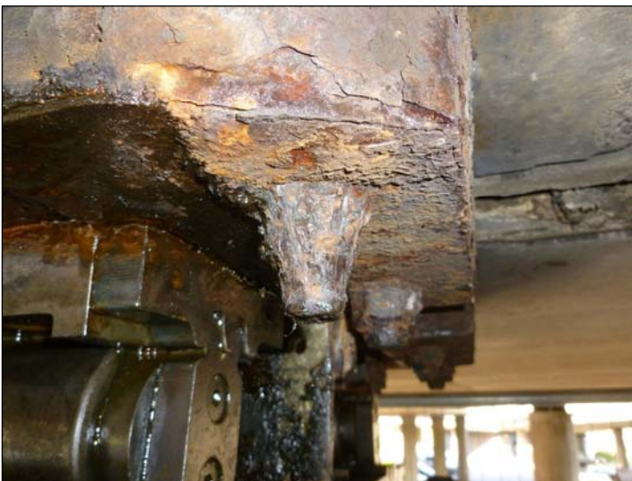
Bearing C2; Significant loss of section to nut of top steel plinth.
