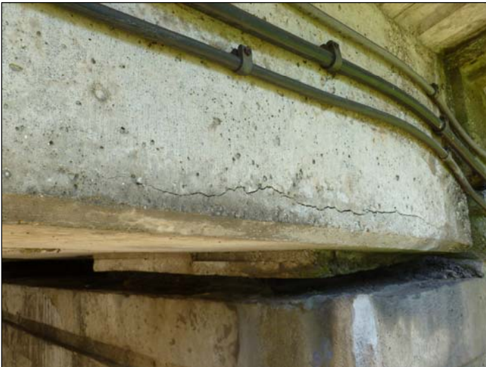
Deck Edge Adjacent to Bearing A; Reinforcement corrosion crack along deck edge.
