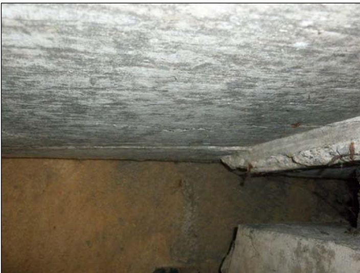
Between Bearings C & D; Delaminated concrete to the deck soffit adjacent to joint.
