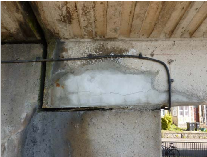
Above Bearing E; Failed repair to the south end of the deck at abutment.
