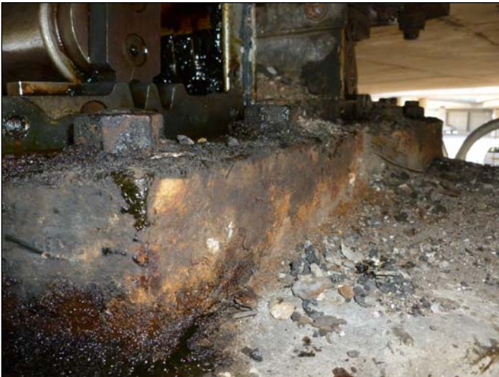
Bearing B2; Delamination to bottom steel plinth.
