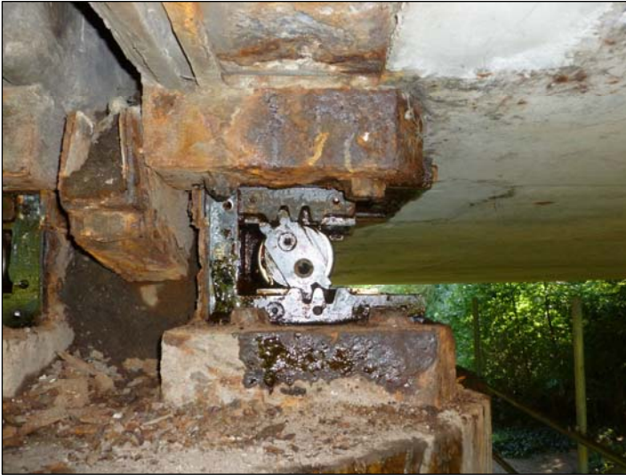
Bearing D1; This is the largest rotation to a guide on the structure.
