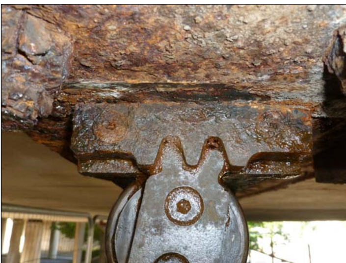
Bearing C1 Significant corrosion over surface of guide rack and some pitting and light surface corrosion to higher level of roller guide.
