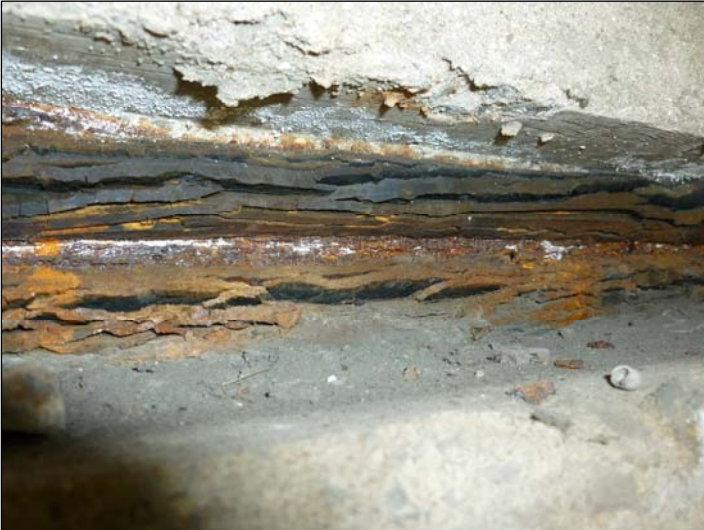
Bearing C; Cracking to elastomer and corroding steel plates.
