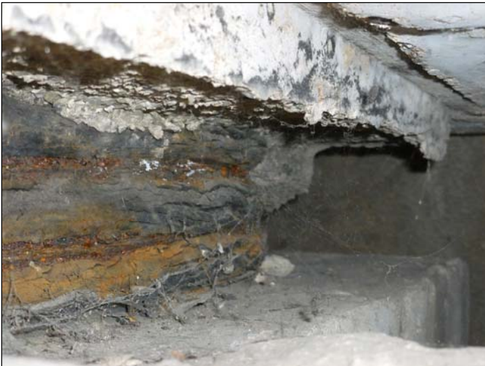
Bearing C; Splitting and bulging of the elastomer and exposed corroding steel plates.
