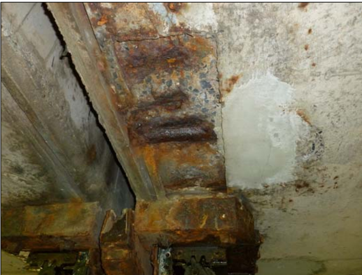
Bearing D2; Failed repair to deck soffit adjacent to joint exposing reinforcement to the south of bearing D2.
