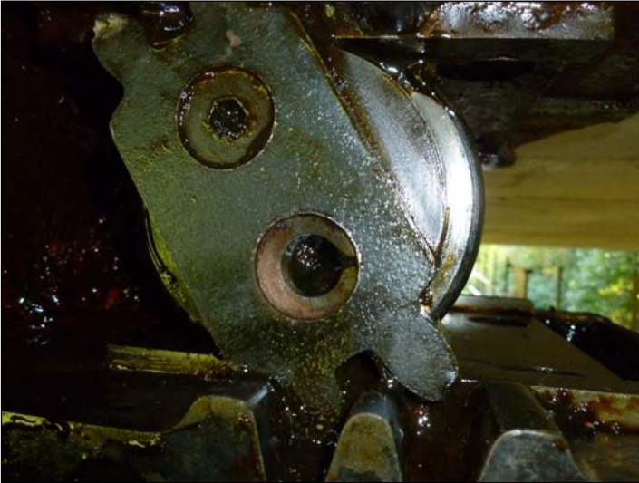
Bearing D2, Missing fixing to south guide of bearing. The missing fixing was not found during removal of grease so it can be assumed that there was never a fixing attached.
