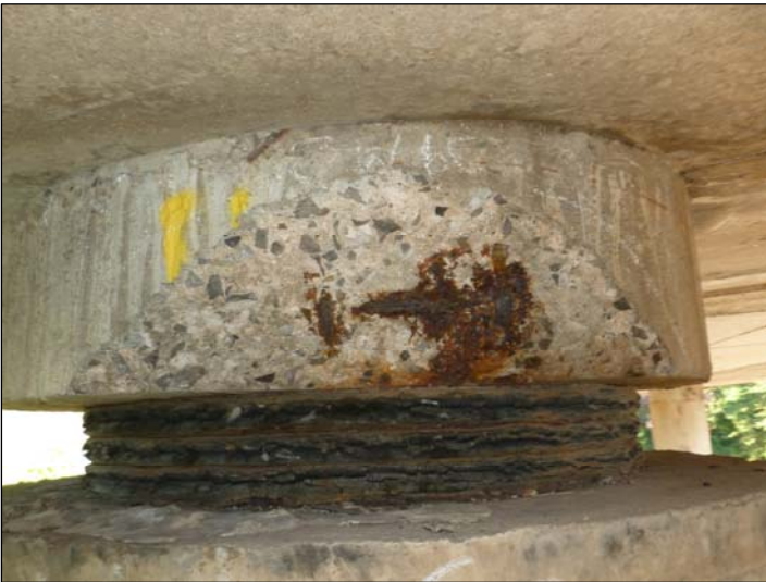
Bearing C; Spalled concrete and exposed corroding reinforcement to top plinth.
