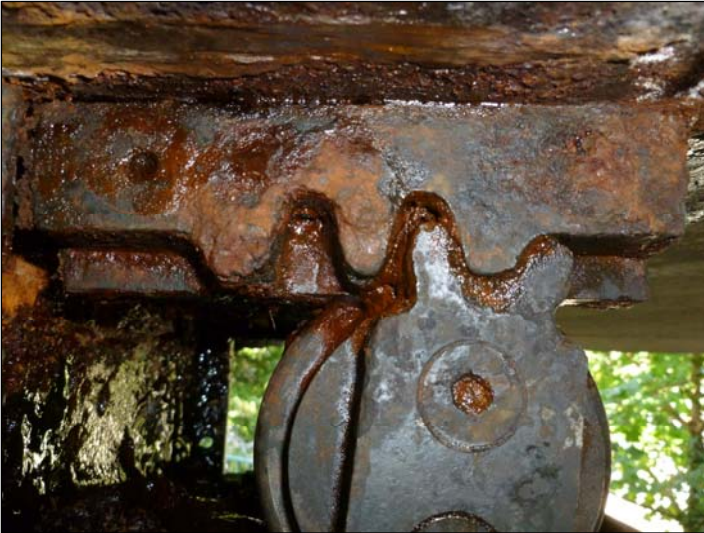
Bearing A2; Again, corrosion to guide rack and roller but also the guide appears to have been set on the wrong tooth.
