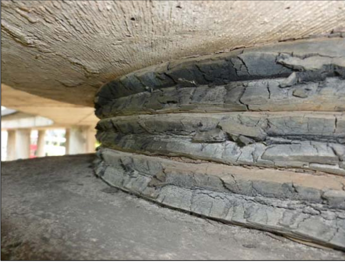
Bearing C; Splitting of elastomer
