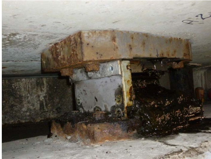
Bearing B before Full Removal of Grease Box
