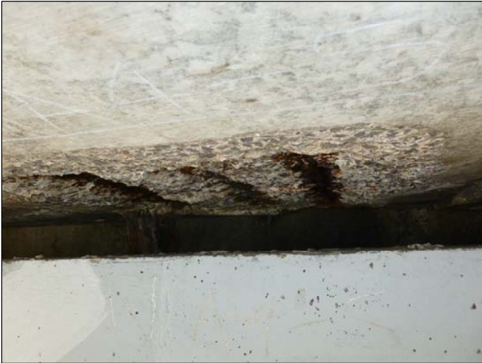
Between Bearings D & E; Spalled concrete exposing corroded reinforcement to the deck soffit.
