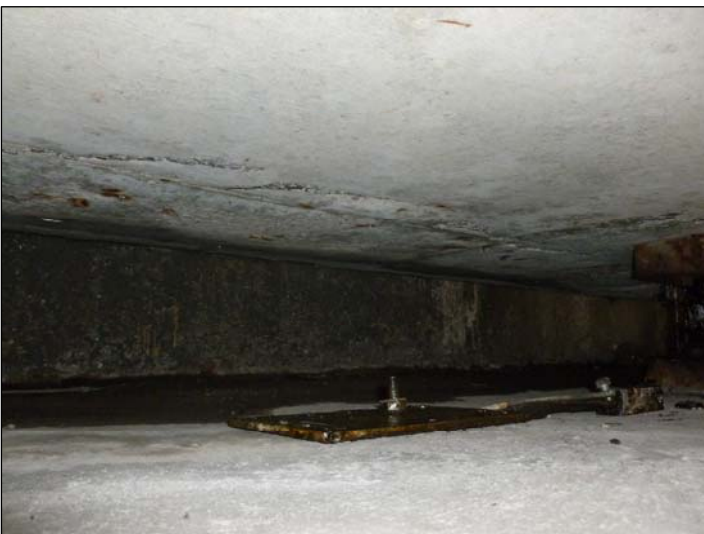
Adjacent to Bearing B; There is delaminated concrete to the deck soffit adjacent to the deck edge.
