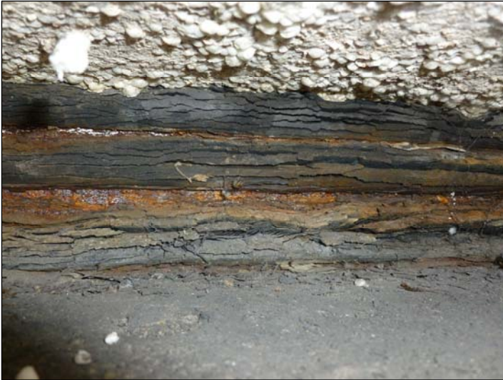
Bearing A; Splitting of the elastomer and exposed corroding steel plates.
