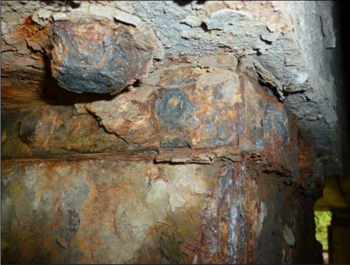
Bearing A2; Delamination of steel and corrosion to bolts made it difficult to remove the sides of the grease boxes.
