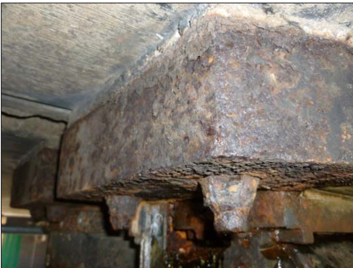
Bearing A2 Heavy corrosion to steel plinths and loss of section to nuts.
