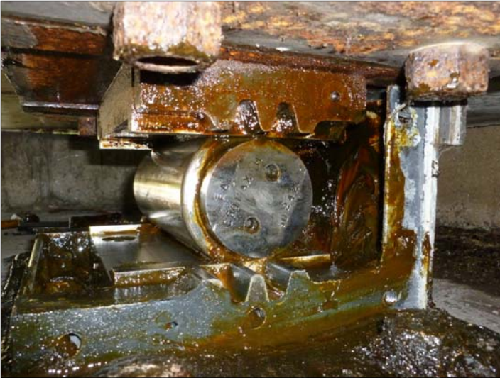
Bearing A; End of roller bearing with roller guide removed for ultrasonic testing which is in good condition.
