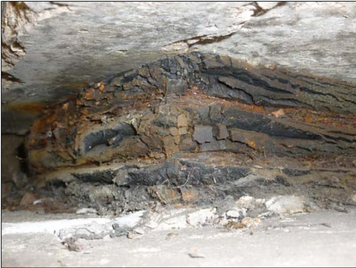
Bearing A; Deterioration to the elastomer and corrosion to exposed steel plates.
