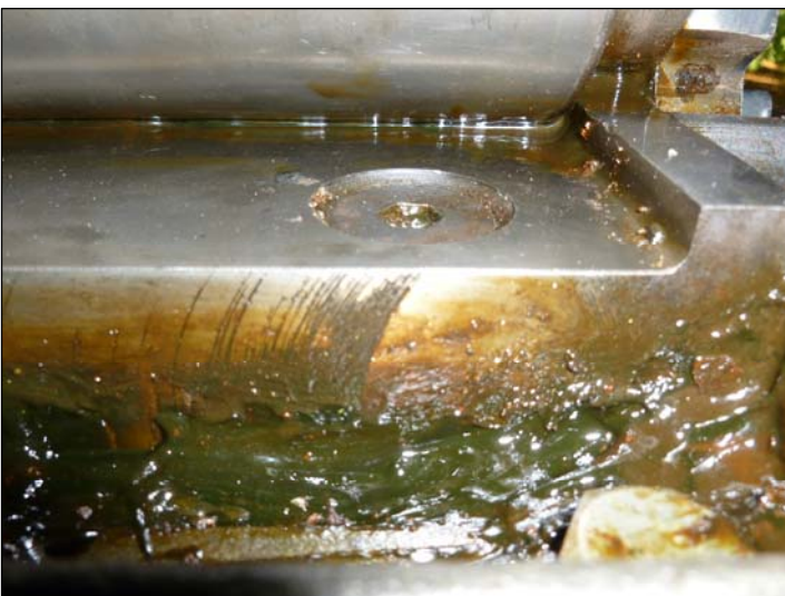
Bearing B2; Typical condition of base plate and base plate fixings.
