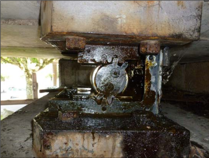
Bearing A; The roller guide has been set to wrong position.
