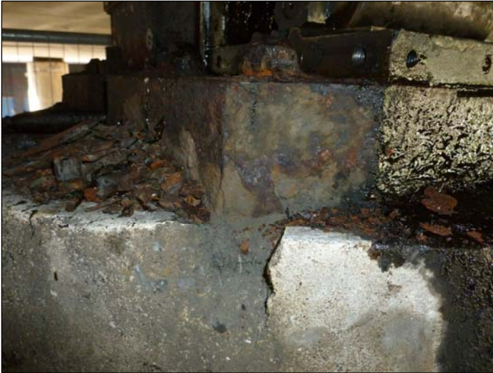
Bearing A2; Small spall in top of column adjacent to corner of steel plinth.
