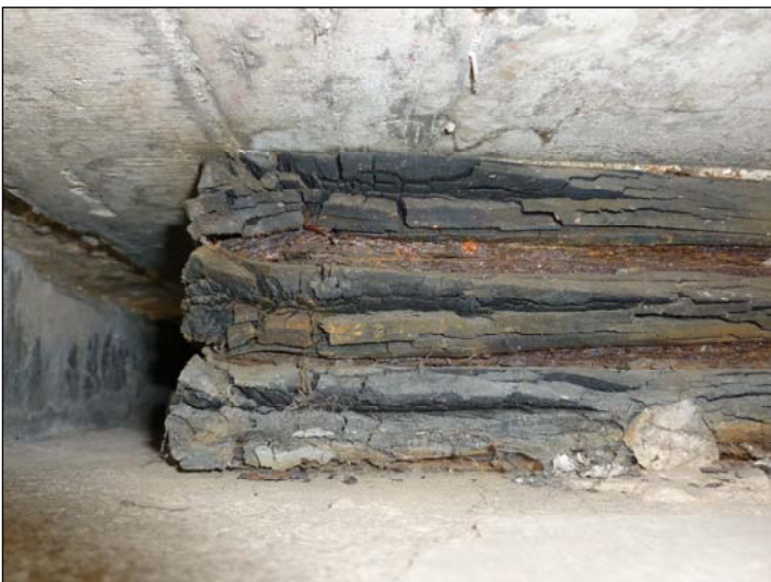
Bearing E; Deterioration to the elastomer and corrosion to exposed steel plates.
