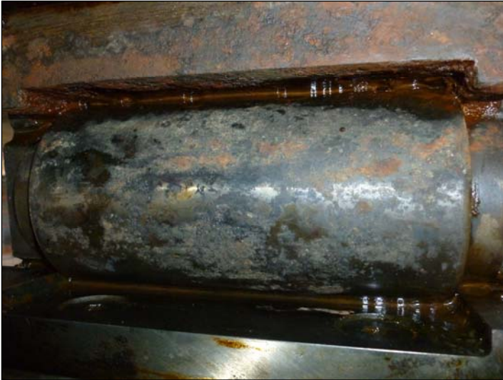
Bearing A2; Light to moderate surface corrosion over 80% of surface of roller.
