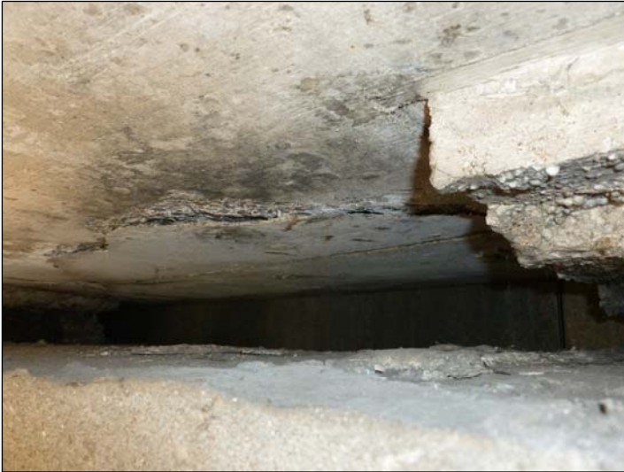
Between Bearings C & D; Further delaminating concrete to the deck soffit adjacent to the deck edge.
