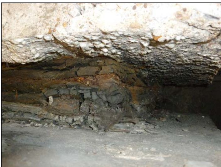
Bearing E; The elastomerics are splitting and exposing corroded steel plates which are themselves delaminating.
