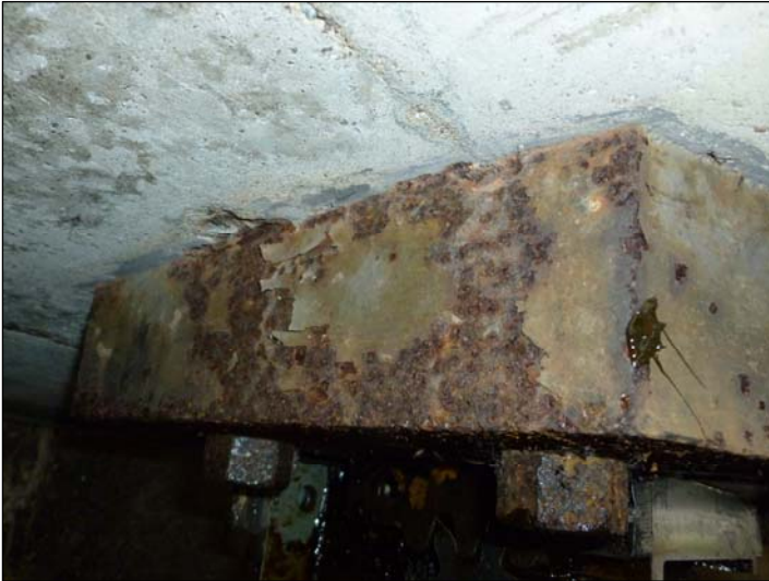
Bearing B; Corrosion to steel top plinth with flaking paintwork and pitting to surface.
